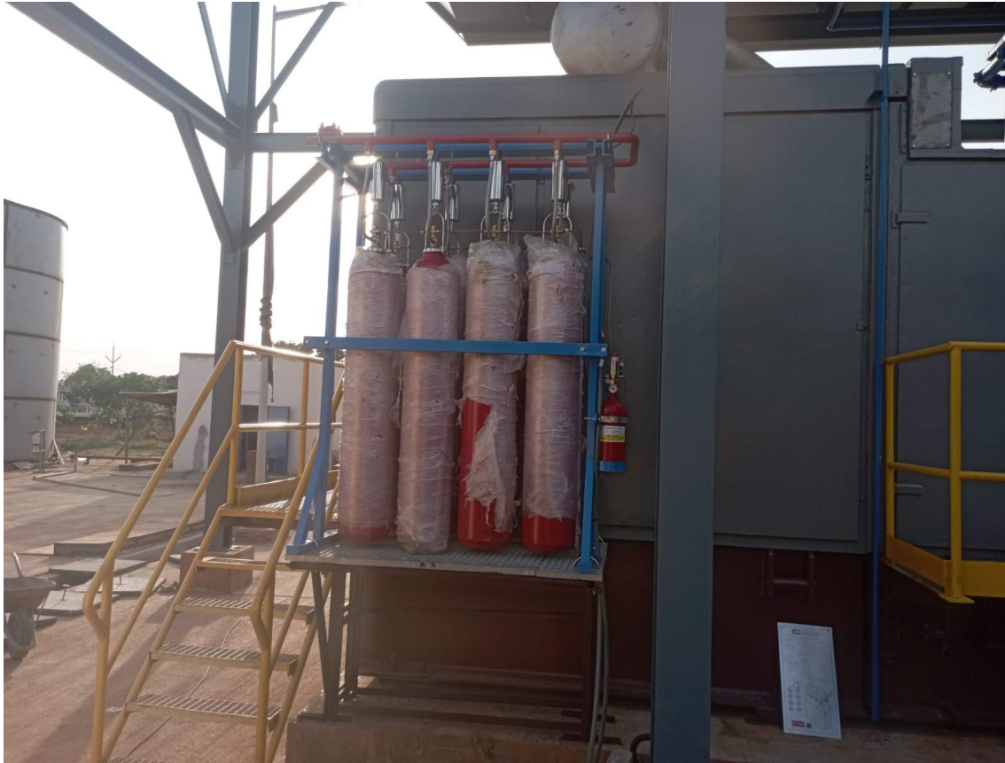
Power station uses CO 2 gas fire suppression system
